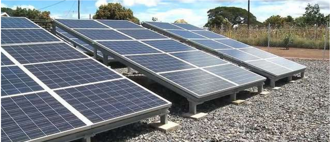
Solar Panels in Zambian Village Credit: UNIDO
